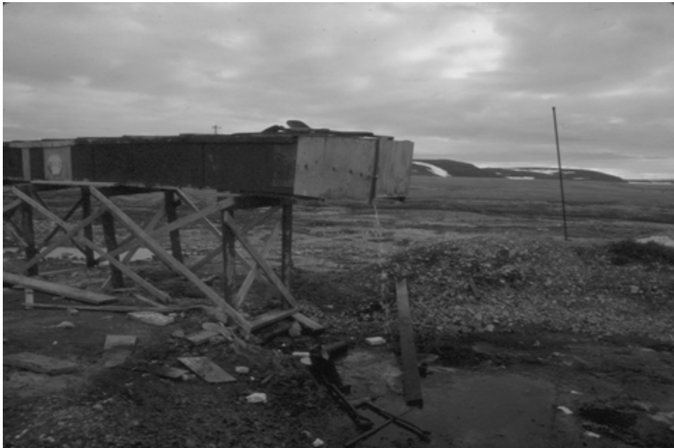
Fig. 11.22 This utilidor system, which was recently dismantled, is releasing sewage and gray water from the Resolute Bay (Cornwallis Island), North Base into a series of streams and ponds. The effluent ultimately reaches Meretta Lake, about 1.6 km downstream.
